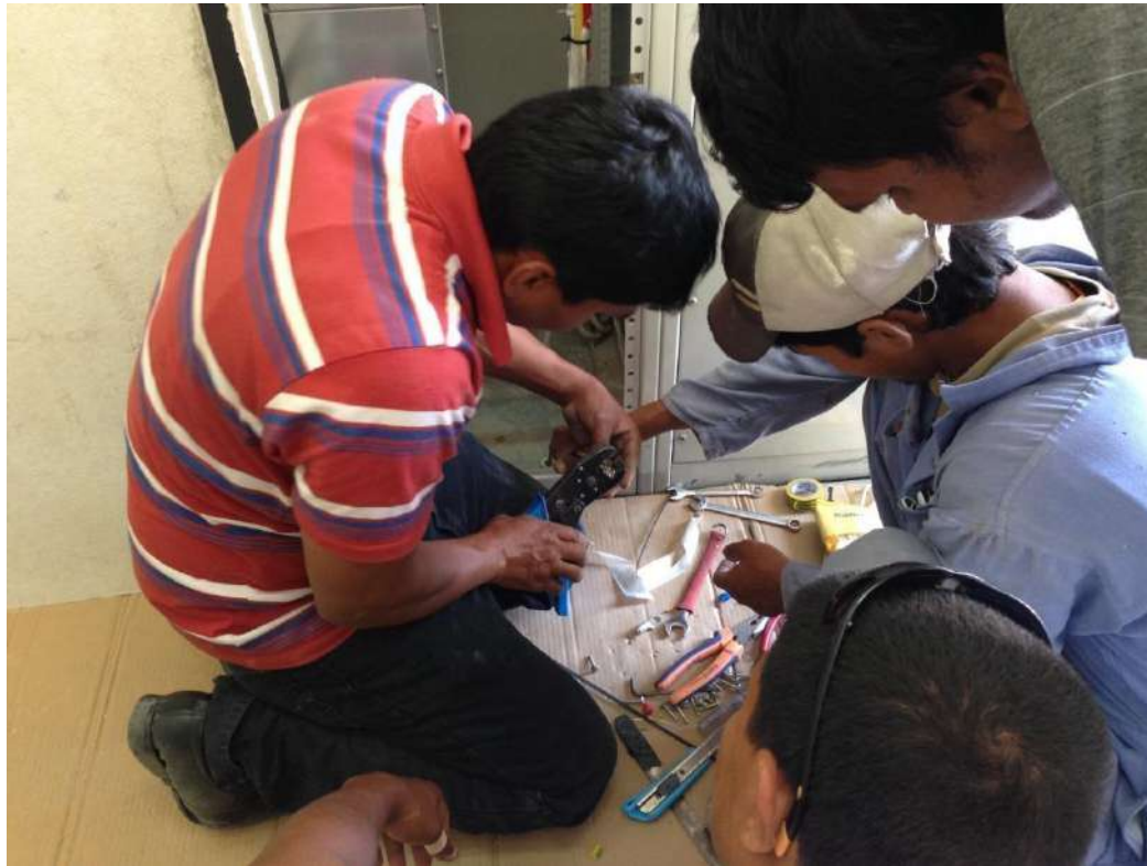
New staff training and offices for Amiri Guards at HGH parking building (Electrical connection in MV room)
