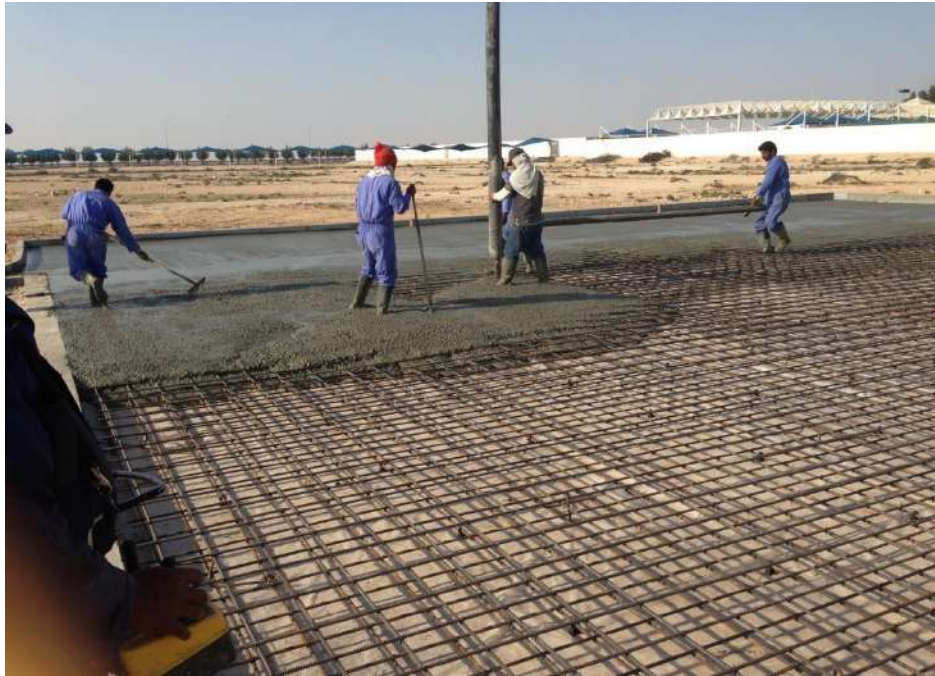
Helipad and Connecting Road at Al Khore Hospital (RC slab for Helipad)
