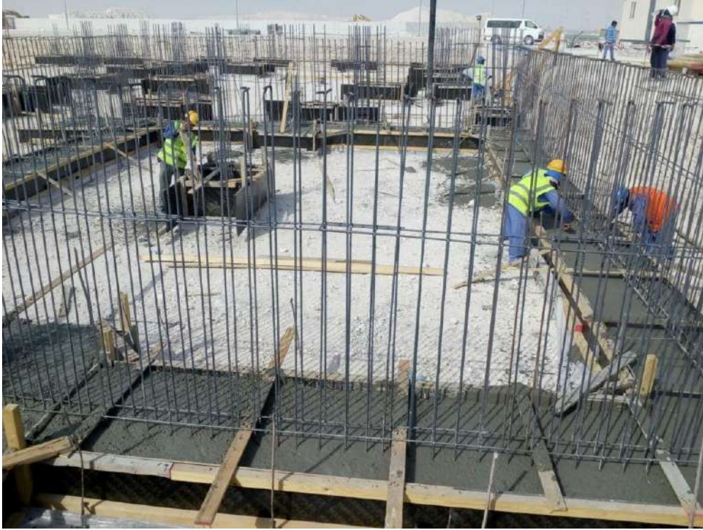
Construction of Warehouses, Accommodation, Offices, Showrooms for Alat Trading Heavy Equipment Co. - Foundation Work
